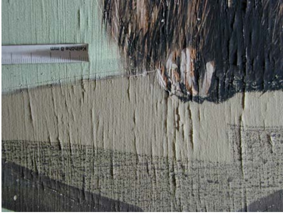
Figure 9 Tenting paint layer.
